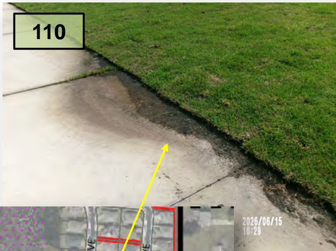
110.Enclave – boardwalk area: Irrigation leak present and requires repair. (Pic 110)
